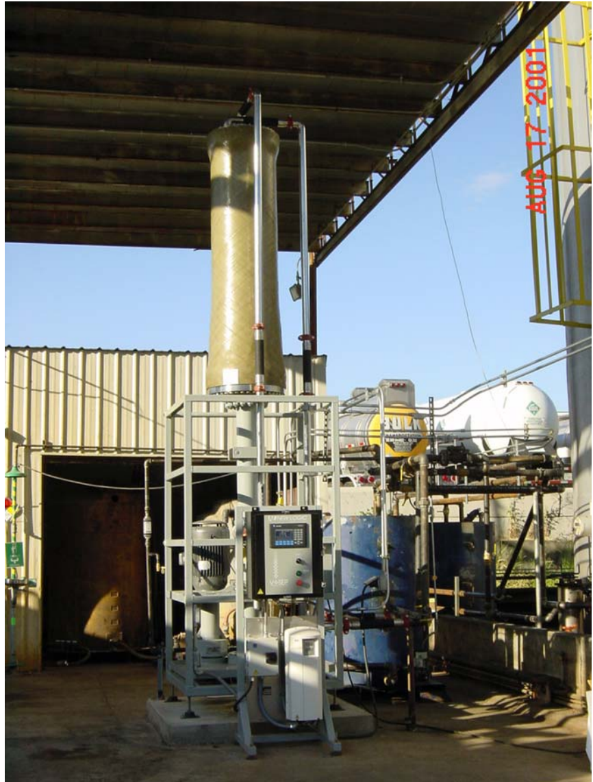
One V◇SEP Unit installed, Footprint is about 16SF
