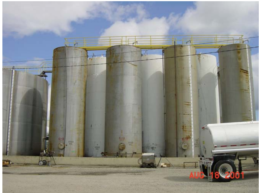
Fuel Storage Tank Farm
