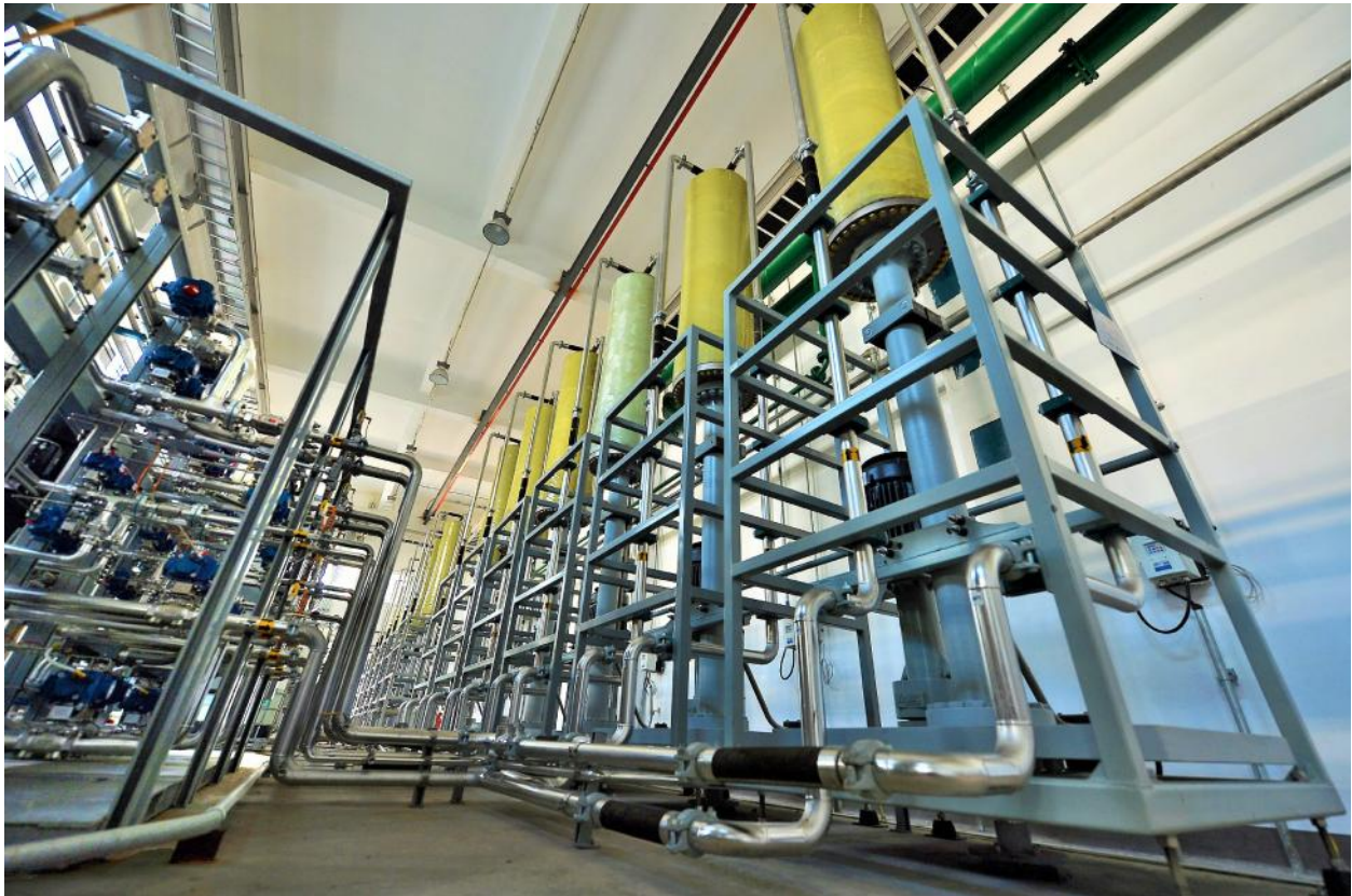
VSEP RO Reject Installation, Inner Mongolia, PRC / Photo Courtesy Edwin Wong
