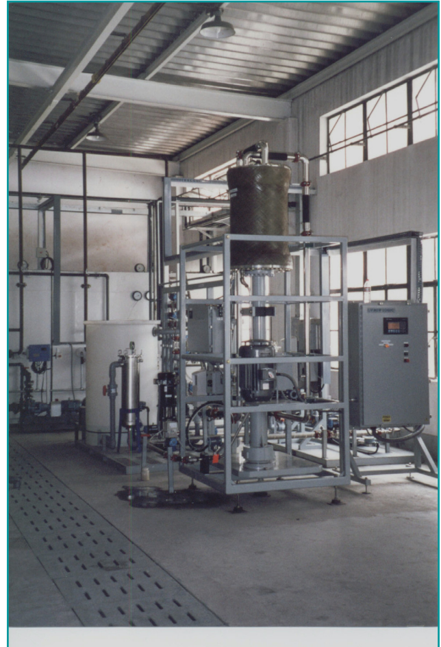
V◇SEP Membrane System installed at a major manufacturing facility for oily water filtration.
