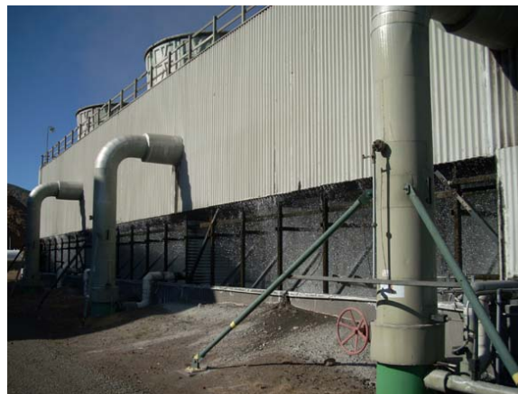
Northern California Power Plant Cooling Towers
