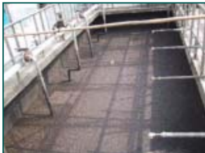
Concentrate Holding Tank
