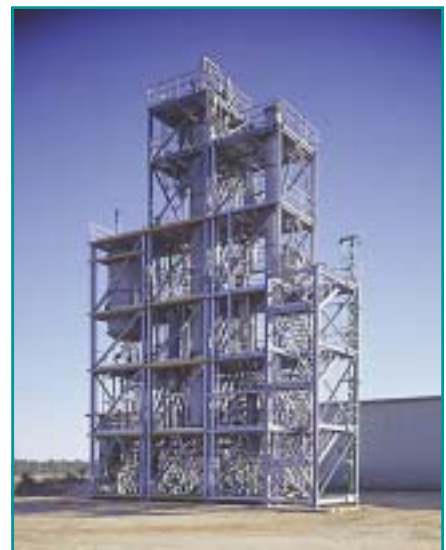
Distillation Column for Glycol Deicing Fluid Recovery
