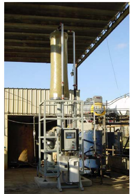
VSEP installed for Used Crankcase Oil Filtration & Recycling
