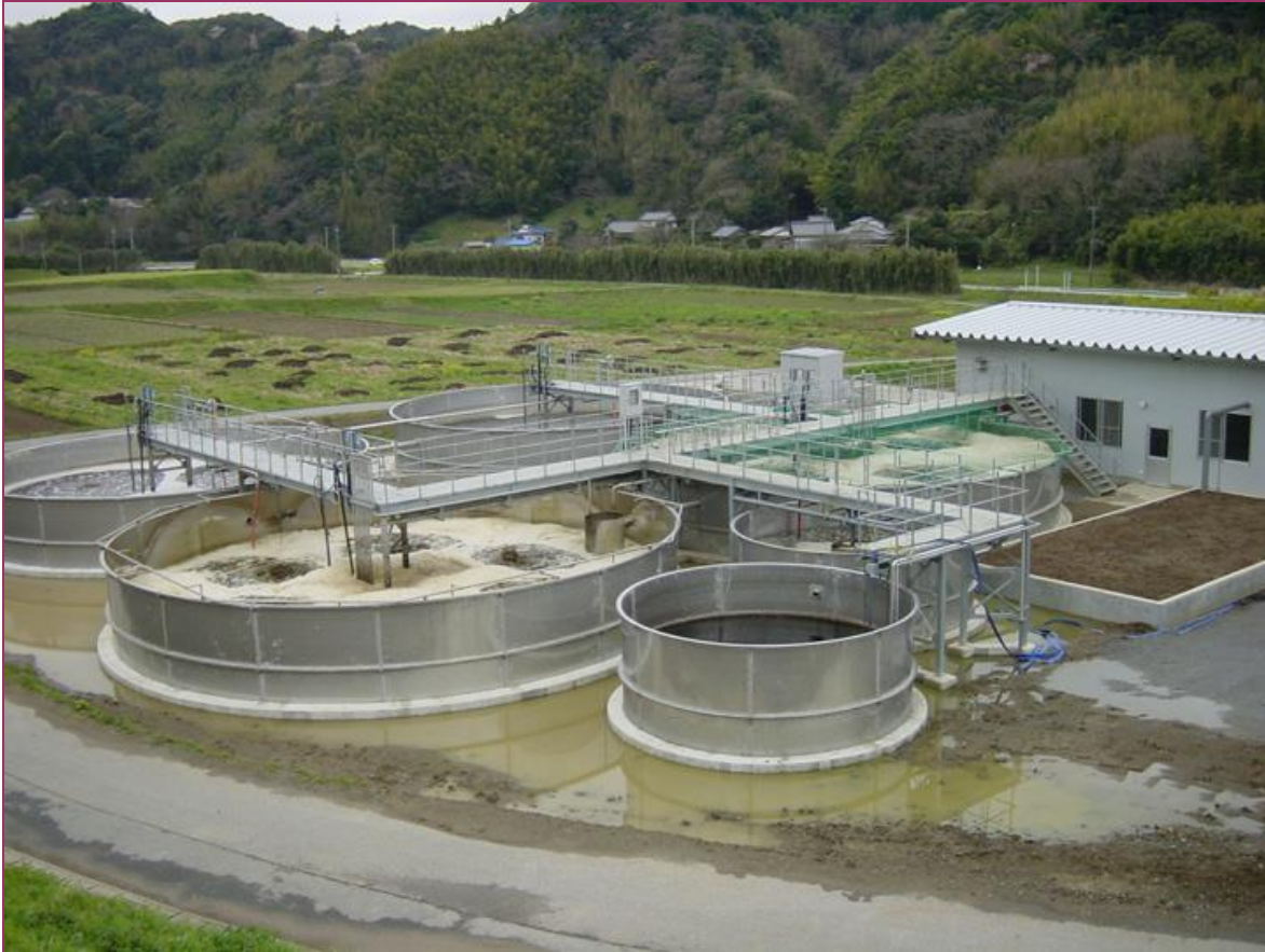
Typical Outdoor Aerobic Digester (Japan)
